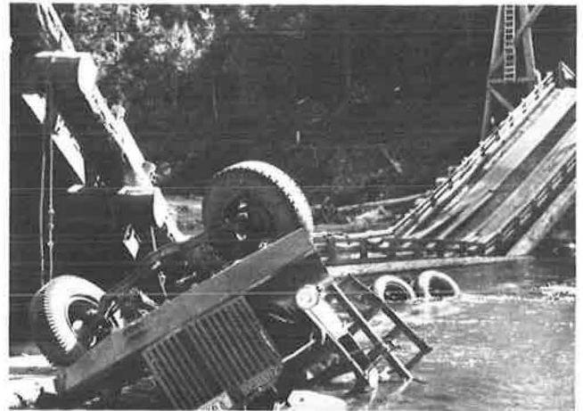
Figure 1. Collapsed log bridge in Oregon.
