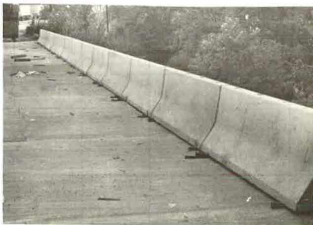
Figure 9. Modular precast parapets positioned on shims prior to being anchored in place with grout.
