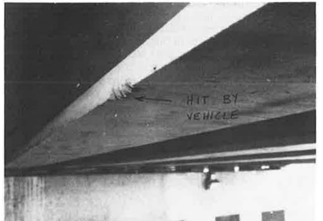
Figure 13. Notch caused by impact from truck.
