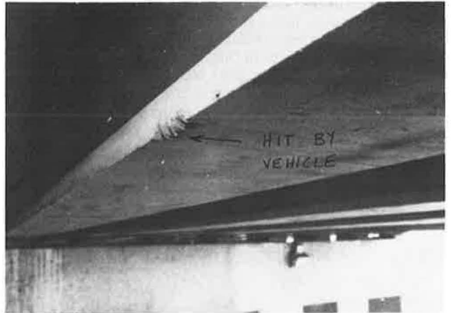
Figure 13. Notch caused by impact from truck.
