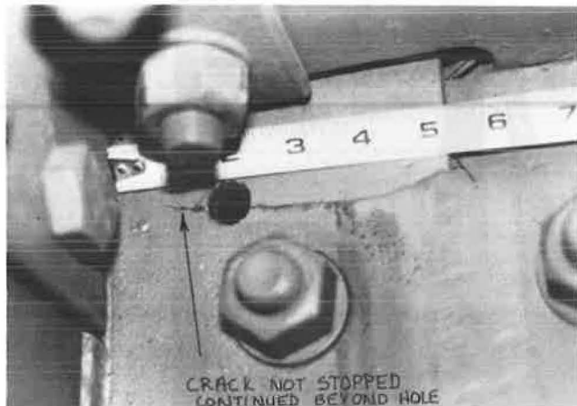
Figure 16. Hole that did not contain crack tip.
