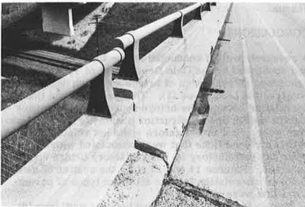
Figure 8. Differential displacement in curb and railing.
