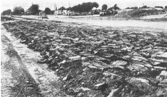
Figure 2. Overall view of section of ripped-up pavement.
