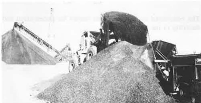
Figure 5. Loading crushed, salvaged bituminous material onto conveyor, which feeds pug-mill stockpile in background.
