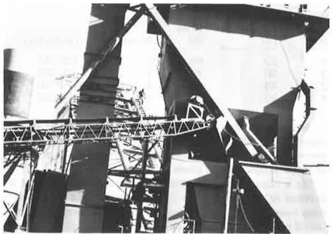
Figure 6. Point at plant where conveyor feeds cold salvaged bituminous material into pug mill.
