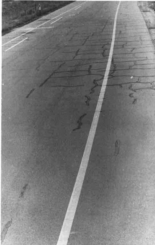
Figure 2. Two adjoining sections, cracked and uncracked; the cracks sealed with bitumen emulsion.
