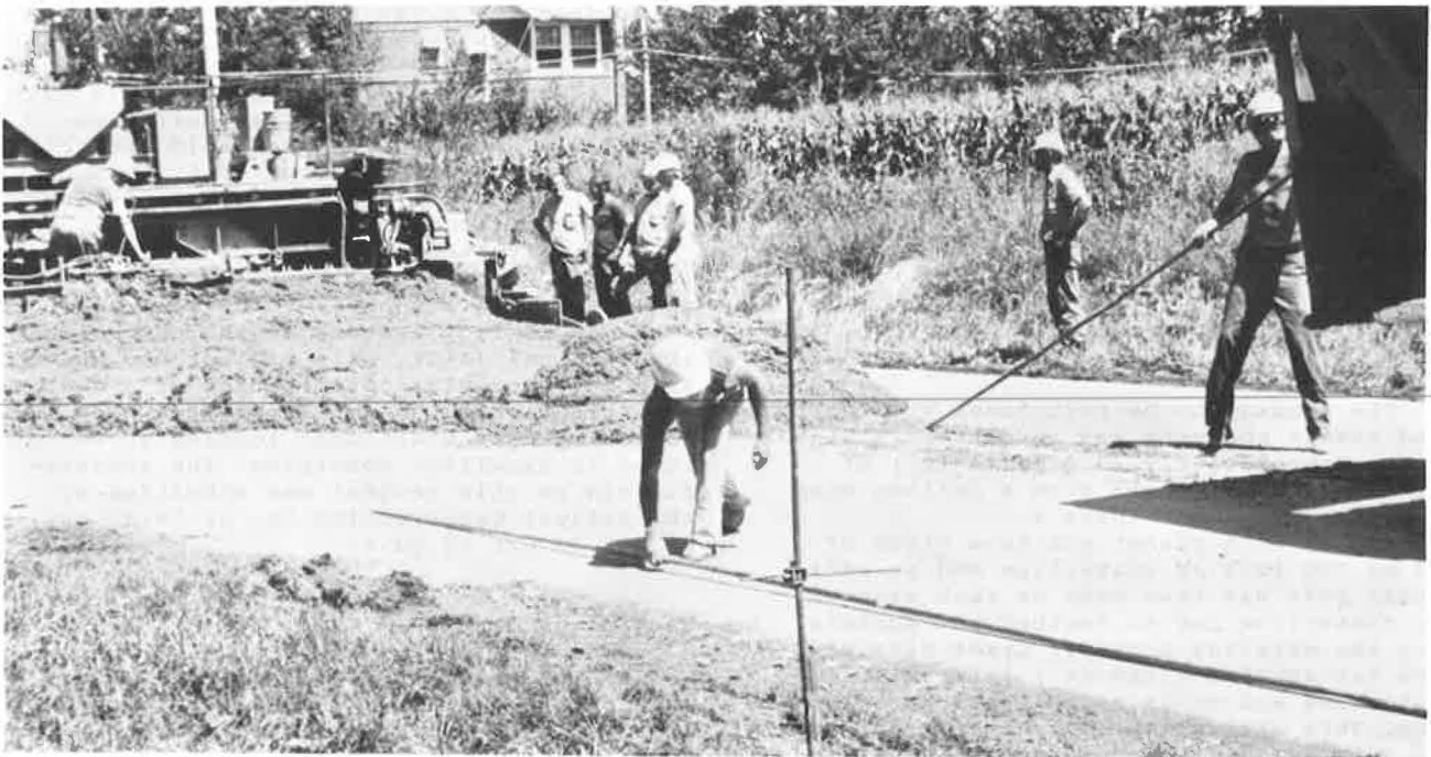
Figure 6. Depicts the entire pavement train including the process of concrete delivery. Note stringline placement.
