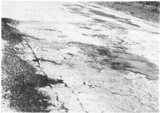
Figure 10. General condition of the existing asphaltic concrete pavement at the time of overlay with portland cement concrete.
