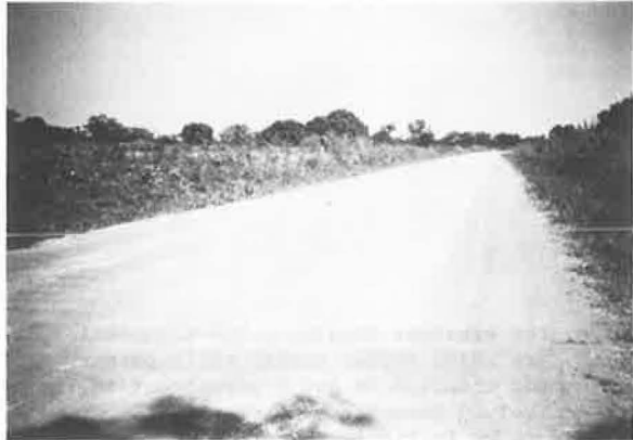
Condition 3 - surface deterioration.
