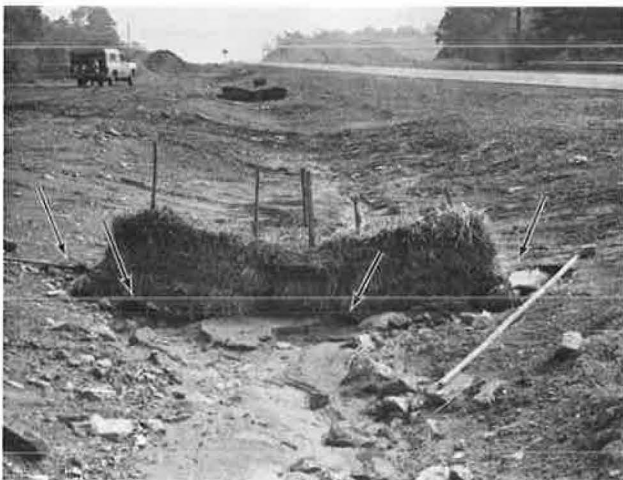
Figure 1. Straw barrier placed by a contractor; arrows indicate failure by undercutting and end flow.
