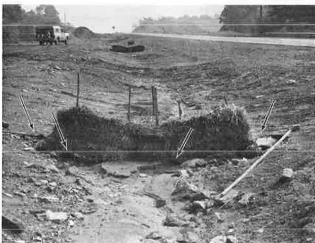
Figure 1. Straw barrier placed by a contractor; arrows indicate failure by undercutting and end flow.
