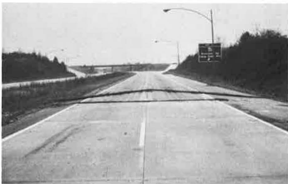
Figure 5. Georgia test site showing cutoff trench, water diversion, and part of section G1.
