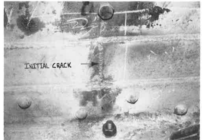
Figure 15. Crack propagated into the web.
