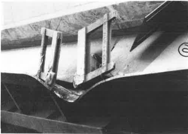
Figure 21. Damage caused by backhoe.
