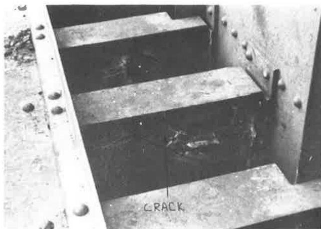
Figure 23. Crack caused by torsional fatigue.
