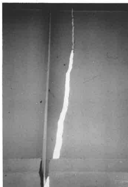
Figure 11. Crack becoming a fracture.
