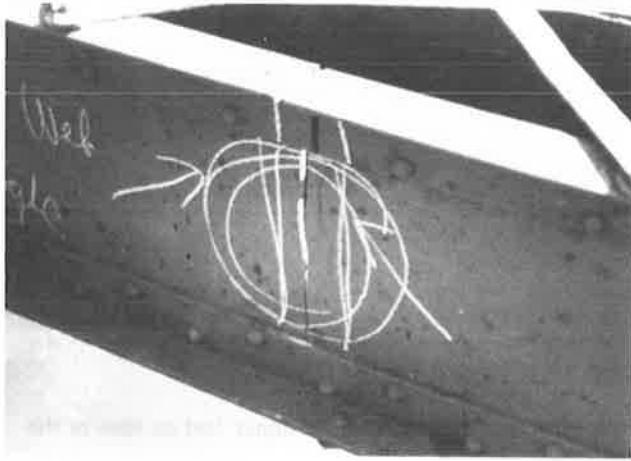
Figure 2. Cracked chord member.
