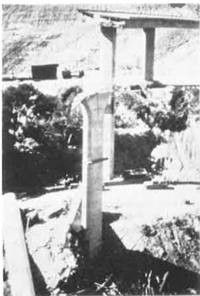
Figure 7. A bridge collapsed by the San Fernando earthquake.
