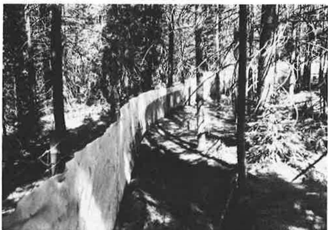
Figure 3. Filter-fence sediment trap.
