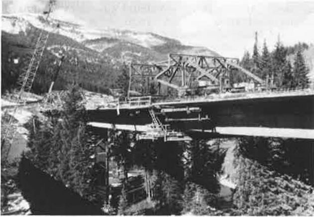
Figure 8. Closure pour after removal of form travelers from other side of bridge: bridge AM.
