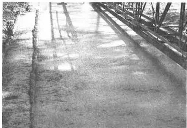
Figure 4. Variable concrete pulling in lower part and flowing in upper part.
