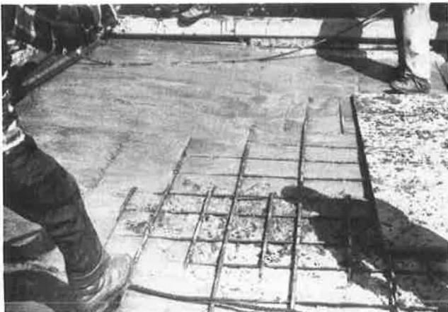
Figure 11. Super-water-reduced concrete flowing out of control.
