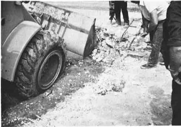
Figure 12. Equipment damage to subbase and subgrade.
