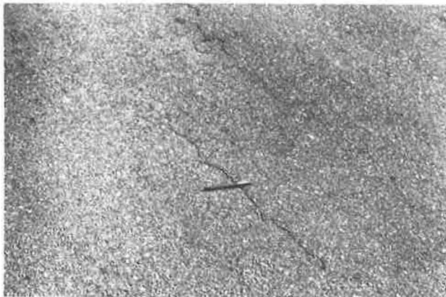
Figure 3. Longitudinal crack in littercrete section.
