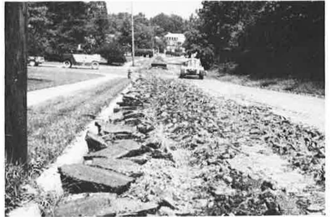
Figure 3. Old mat broken up and recycled into soil-cement on Virginia street project.
