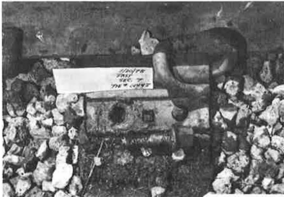
Figure 11. Failed screw spike.
