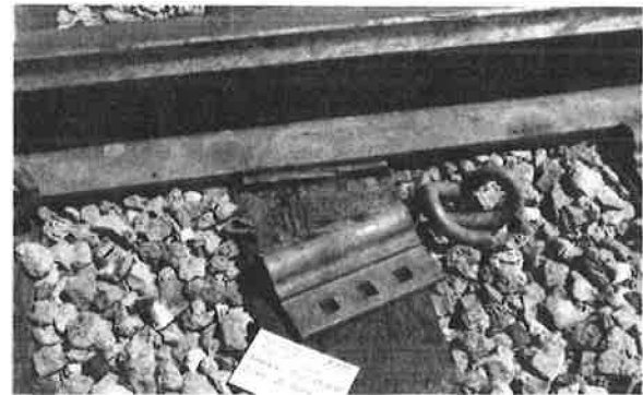
Figure 10. Failure of elastic-clip plate in track.
