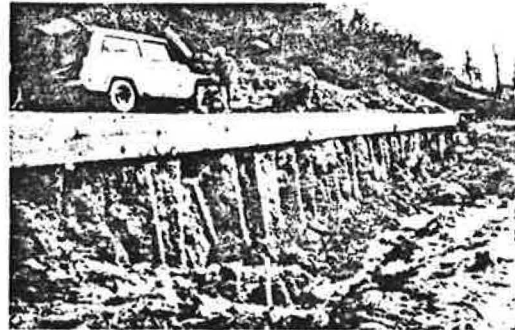
Figure 11. Additional movement that broke slope inclinometer pipes below wall.
