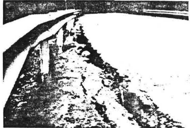
Figure 7. Area west of main failure area.
