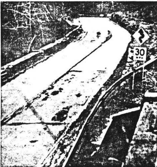
Figure 6. Main failure area.
