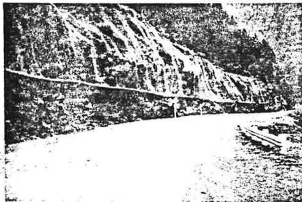
Figure 7. Wire mesh over raveling rock slope to prevent rockfall into grade.
