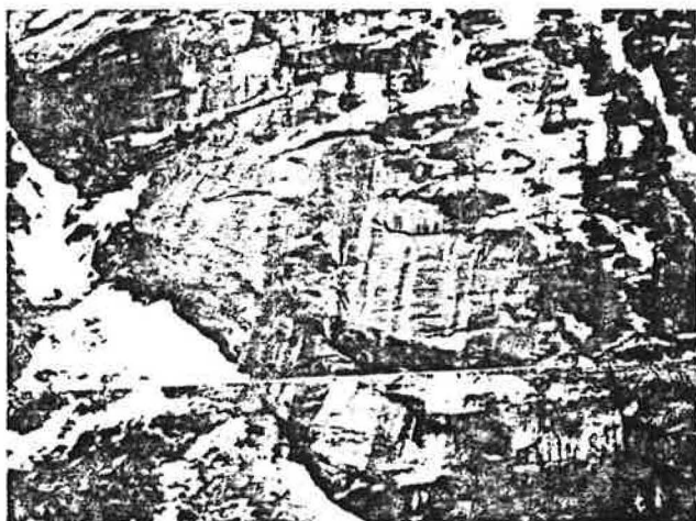
Figure 19. Track threatened by snow and ice sliding from adjacent rock face.
