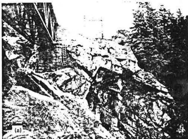
Figure 20. (a) Location where shifting rock block resulted in movement within rock masonry abutment and (b) close-up of anchor cable installed for stabilization.
