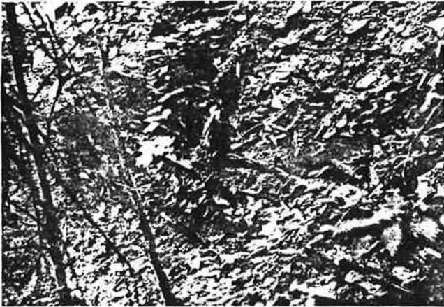
Figure 5. Current condition of timber cribs.
