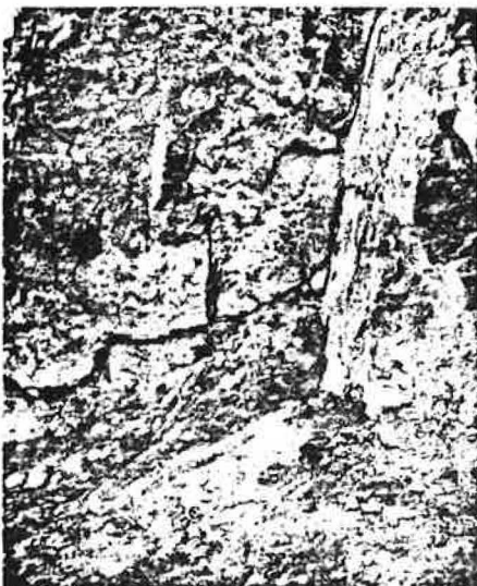
Figure 14. Cause of rockfall that caused train derailment shown in Figure 13.
