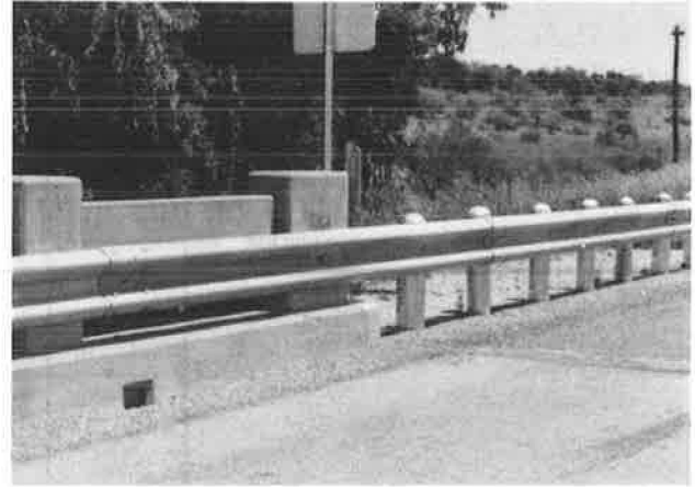
Figure 8. Example of good practice for the transition from approach guardrail to bridge barrier.
