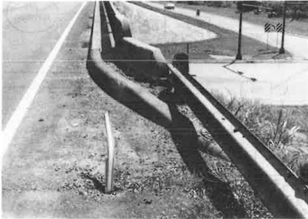
Figure 6. Example of approach guardrail not anchored to bridge railing.
