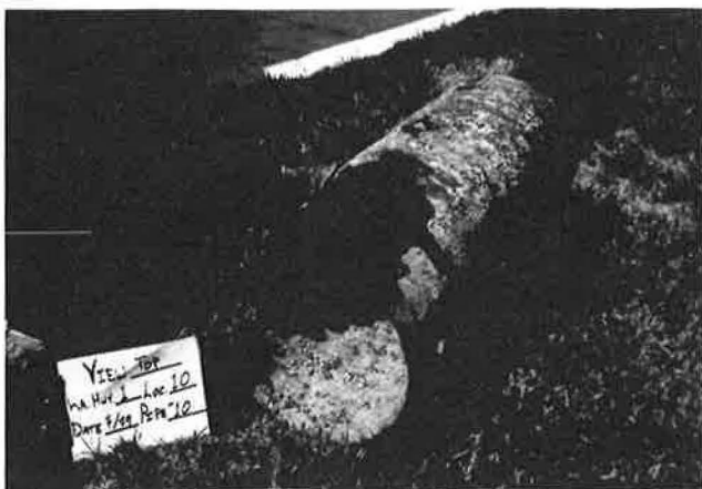
Figure 2. Condition of galvanized-steel culvert in low-electrical-resistivity environment (site 10) after six years.
