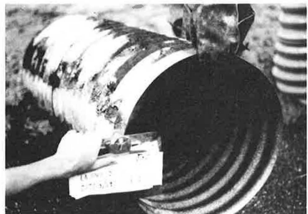
Figure 3. Condition of galvanized-steel culvert in acidic environment (site 4) after six years.
