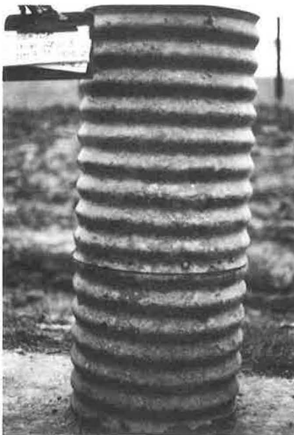
Figure 4. Condition of galvanized-steel culvert in moderate environment (site 5) after six years.
