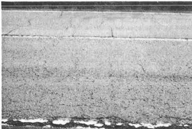
Figure 3. Asphalt T-1 showing effect of C_v on the extent of cracking.
