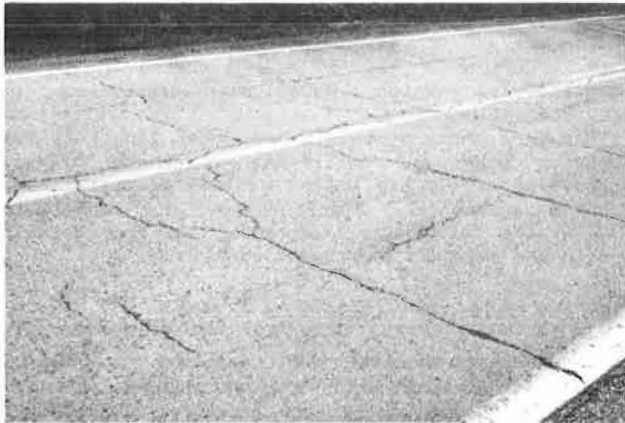
Figure 1. Asphalt T-1 showing transverse and longitudinal cracks in both lanes.
