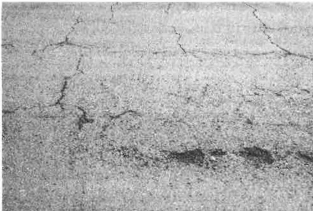
Figure 2. Asphalt T-1 showing block cracking and deterioration.
