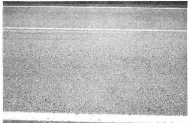
Figure 5. Asphalt T-3 (both lanes).
