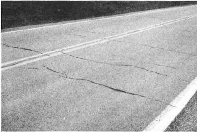
Figure 7. Asphalt T-5 showing well-defined full- and half-width transverse cracks.
