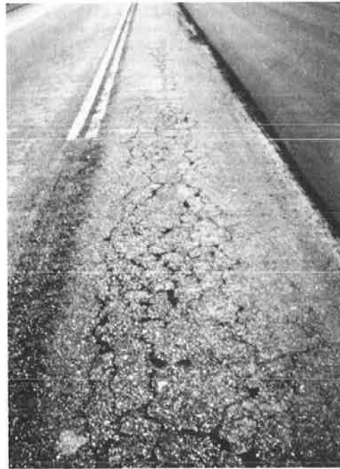
1963 PHOTO OF FATIGUED SECTION (2" AC OVER 8" CRB) WITH RECYCLED SURFACE AND 1" AC BLANKET AT RIGHT, OVERLAY IS STILL IN SERVICE TODAY WITHOUT MAINTENANCE
