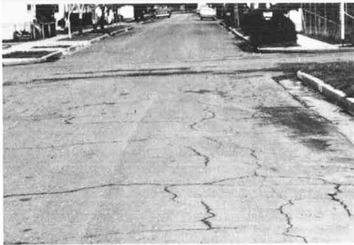
LARGE SHRINKAGE CRACKS FROM EMBRITTLED ASPHALT, ACCUMULATED TRANSMISSION OIL DRIPPINGS, AND WATER DETERIORATION AT GUTTER
