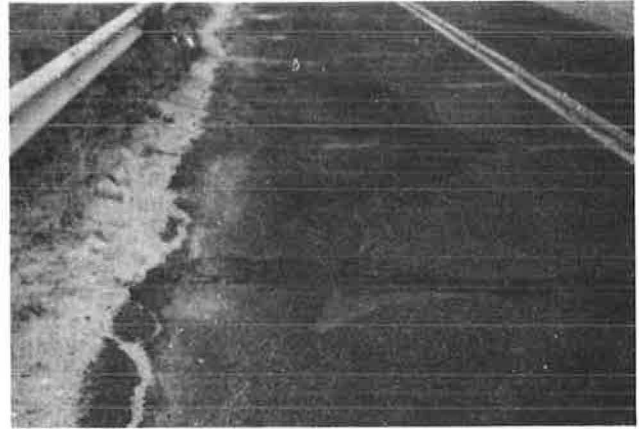
Figure 3. Localized deterioration in the existing pavement.
