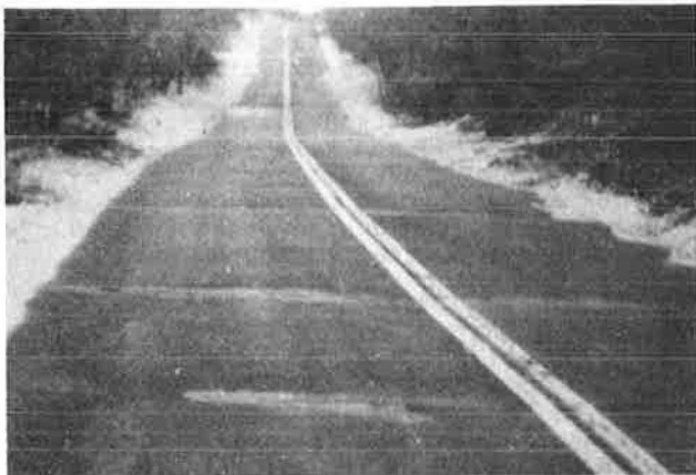
Figure 2. Transverse cracks in the existing pavement.
