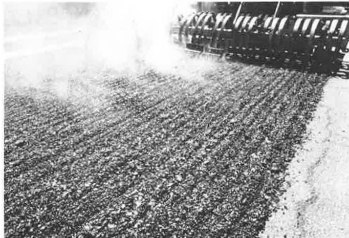
CLOSEUP OF RAKE PENETRATION FROM H.D. SCARIFYER ASSEMBLY PRODUCING 1" SURFACE RECYCLING - NOTE SHRINKAGE CRACK AT RIGHT
