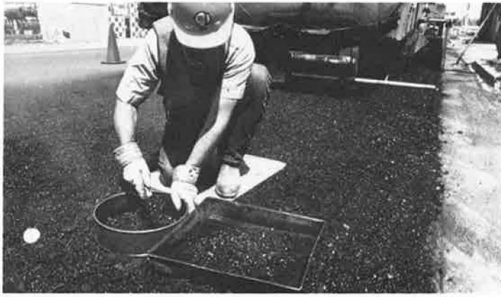
INSPECTOR MEASURES TEMPERATURE AND TAKES SAMPLE OF RECYCLED MATERIAL FRONT OF SCREED
