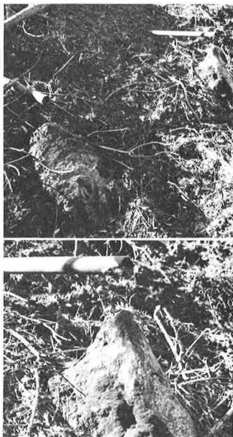
Figure 9. Iron oxide and algae build-up, Nojoqui Grade, 1978: distant view of two drains (top) and close-up of drain at right (bottom).
