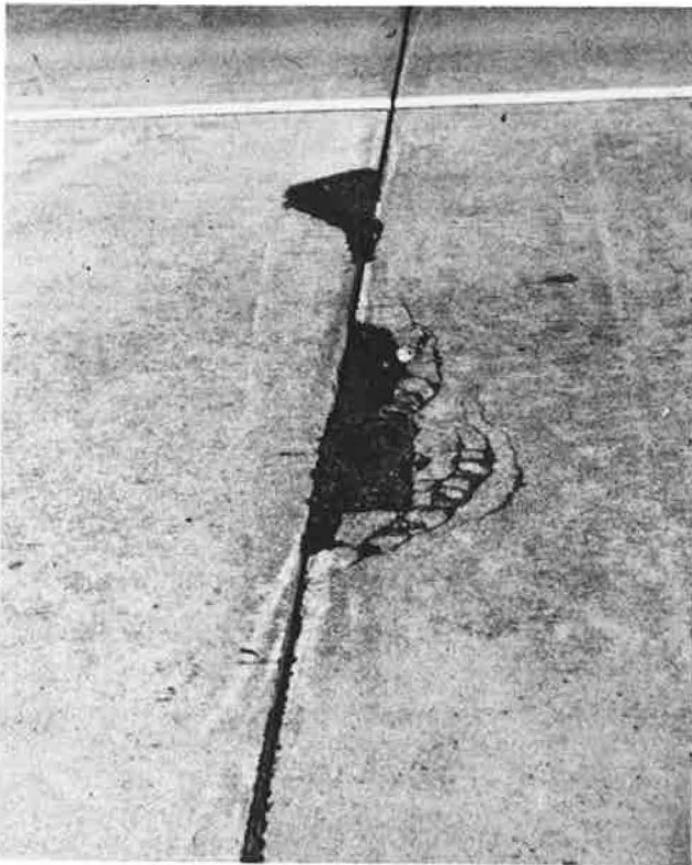
Figure 1. Semicircular spall caused by corrosion of insert.
