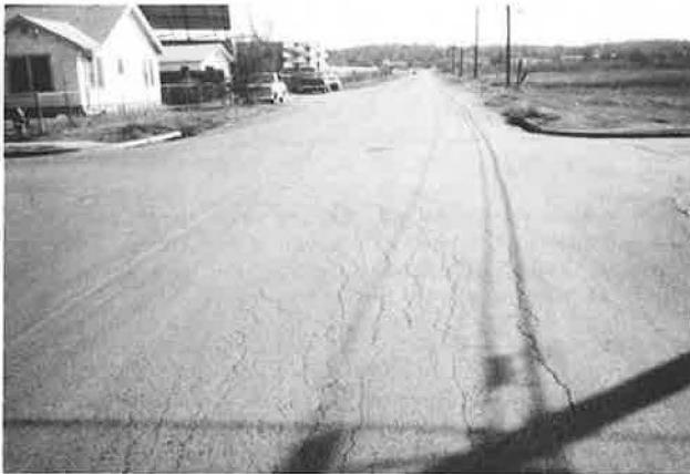
Figure 13. Extensive cracking of pavement on Vargas Street (parallel to and one block from Montopolis Drive).
