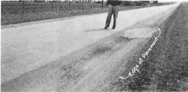
Figure 4. Failures and patching along edges of pavement where crushed conglomerate base material was placed in trench cut in tight clay soil.
