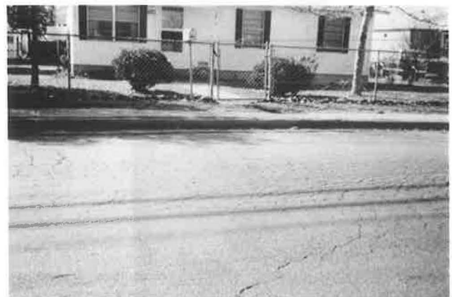
Figure 11. Alligator cracking on Montopolis Drive in east Austin.
