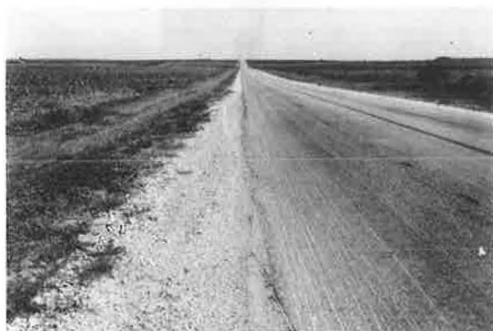
Figure 9. Same section of highway as in Figure 8 after six years.
