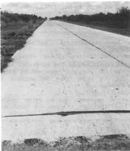
Figure 2. Cracks in pavement when soil fill and natural soil foundation had shrunk.
