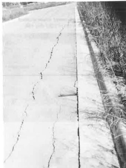
Figure 10. Dry-weather shrinkage cracks on Galen Court, cul-de-sac street in southeast Austin.
