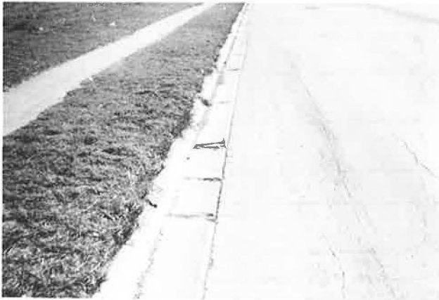
Figure 12. Alligator cracking and possibly some shrinkage cracking on Montopolis Drive.
