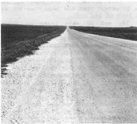
Figure 8. Riding surface after three years of heavy traffic where rain or gravity water moved from base material to ditches.
