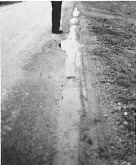
Figure 5. Rainwater in rut in shoulder soil.
