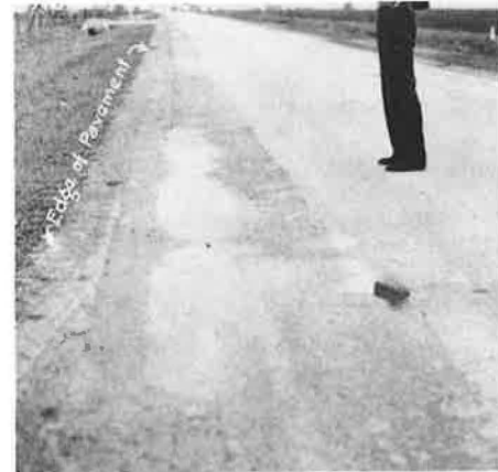
Figure 6. Rainwater in traffic depression caused by movement of underlying clay soil previously overly wetted.
