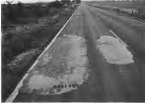
Figure 7. Areas of isolated alligator cracking.
