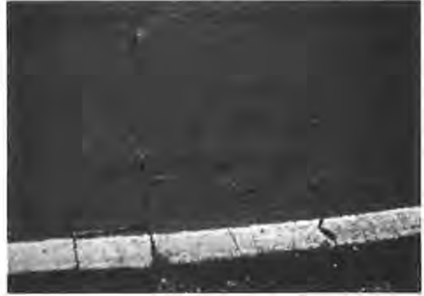
Figure 8. Closeup of alligator cracking in isolated areas.
