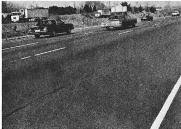
Figure 3. Gouge marks from hard object in surface of open-graded material (southbound, control section).
