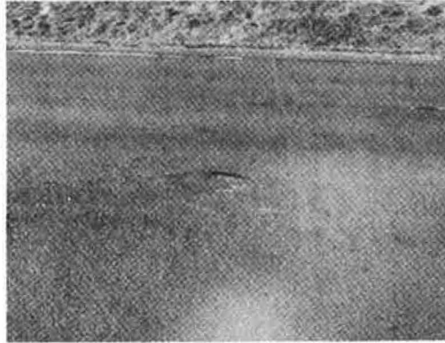
Figure 6. Open-graded material lost beneath thermoplastic line striping during snowplow operations (southbound, control section).
