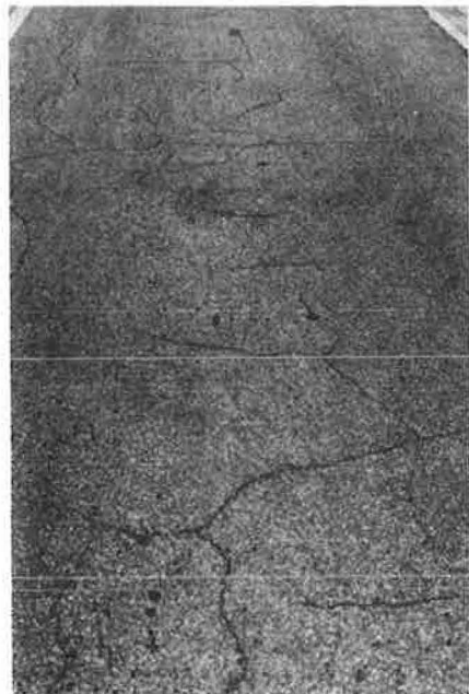
Figure 2. Temperature and age cracks.
