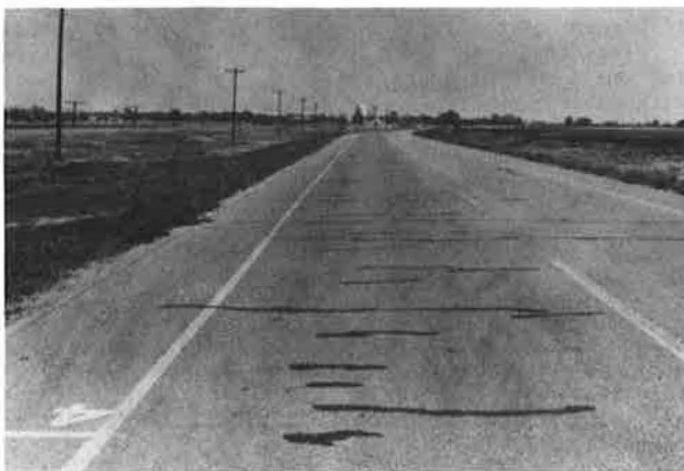
Figure 4. Transverse shrinkage cracking.
