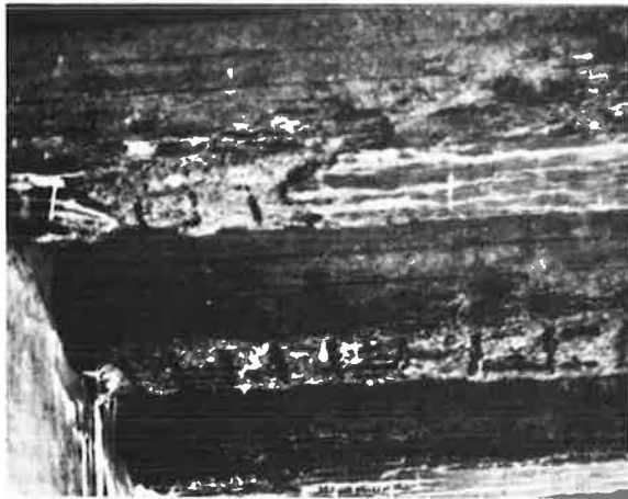
Figure 3. Deterioration of T-beams in bridge 1.
