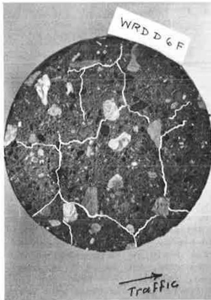
Figure 9. Trace of cracks on polished surface of 4-in-diameter concrete core.
