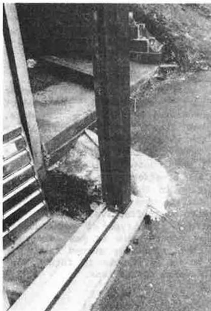
Figure 8. Closeup of support structure, which shows curb, steel H-beam bolted to curb, and 16-gauge U-channel ramset on curb.
