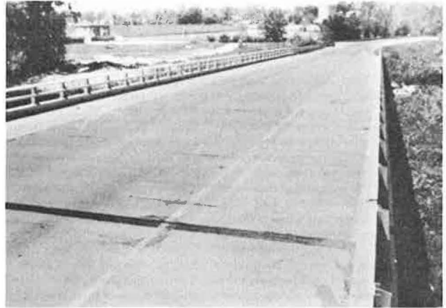
Figure 14. Northbound view of Knightstown bridge deck after 11 years of service.
