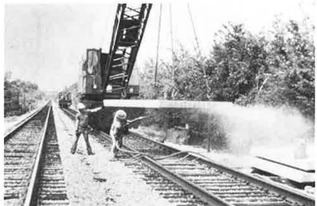
Figure 6. Precast modules are cleaned prior to placement to ensure that epoxy grout will bond.
