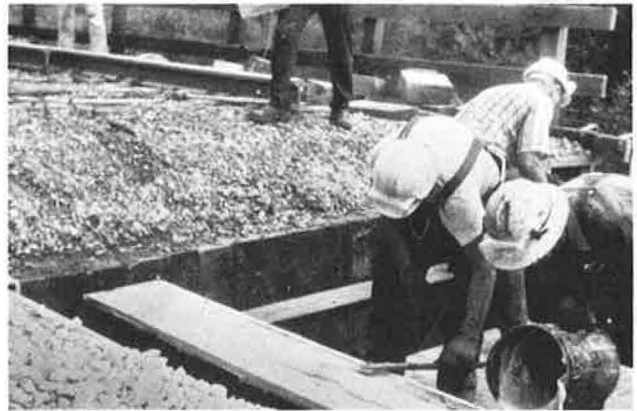
Figure 5. After cleaning, girders were coated with epoxy grout to bond modules to girders.
