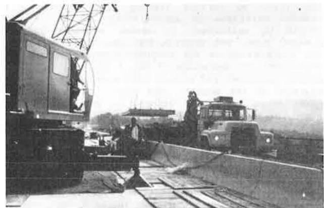
Figure 2. Precast modules are trucked to placement site on operating half of bridge.
