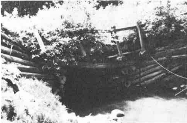
Figure 2. Example of old wood crossing.
