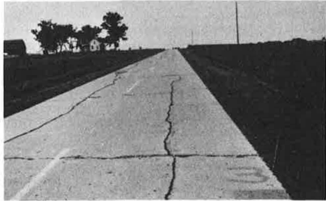
Figure 4. Typical pavement condition of 4.5-in nonreinforced slab in section 3.
