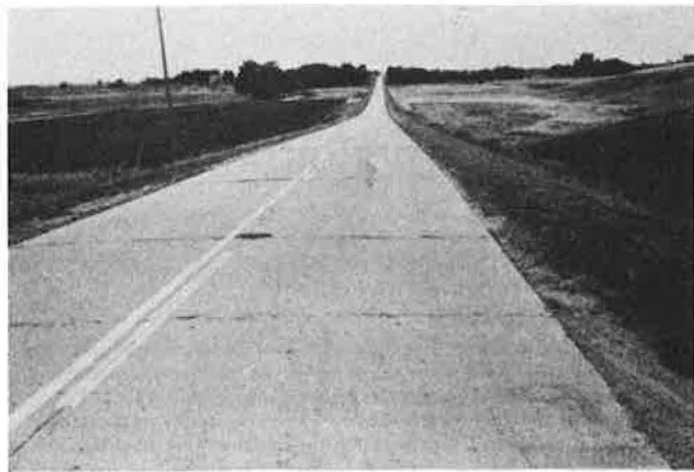
Figure 5. Typical pavement condition of 6-in nonreinforced slab in section 9.
