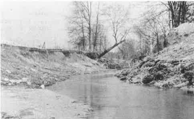
Figure 5. Severe bank erosion caused by degradation on Perry Creek at I-55 near Grenada, Mississippi.
