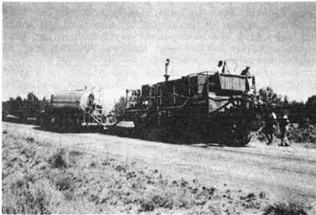
Figure 7. Cold planer pulverizing existing asphalt concrete and adding recycling agent through front-mounted asphalt pump and meter system.
