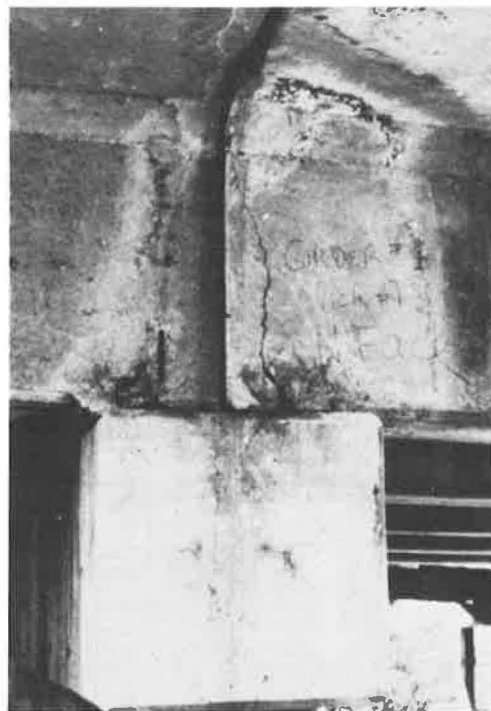
Figure 18. Concrete beam crack.
