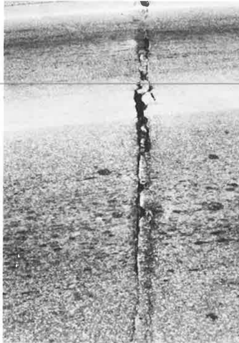
Figure 9. Wearing surface raveling.
