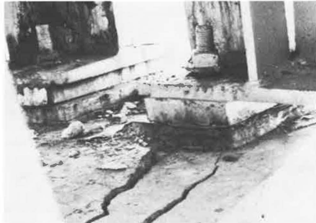
Figure 19. Pier cap crack.
