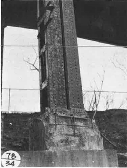
Figure 13. Deteriorated steel and concrete.
