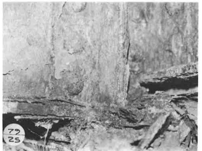
Figure 11. Deteriorated steel member.
