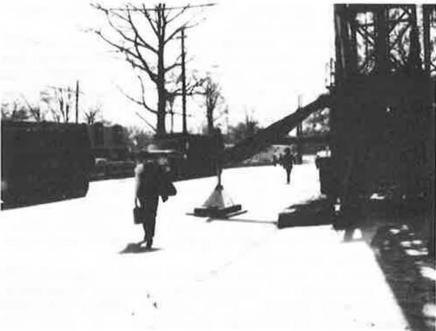
Figure 2. Sidewalk completely blocked by construction equipment; pedestrians forced into traffic lanes.
