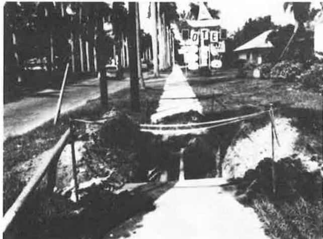
Figure 3. Inadequate protection around utility excavation creates pedestrian safety problem.
