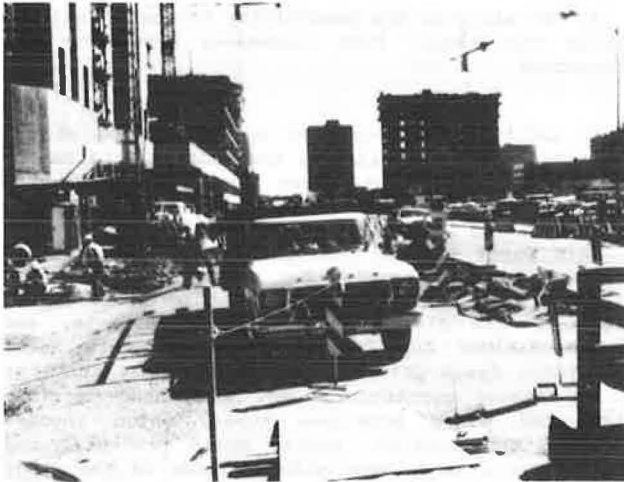
Figure 5. Inadequate delineation of pedestrian pathway and protection results in confusion and discourages use.
