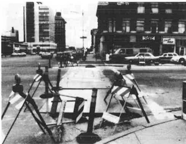
Figure 6. Crosswalk blocked by several devices; no pedestrian information provided.
