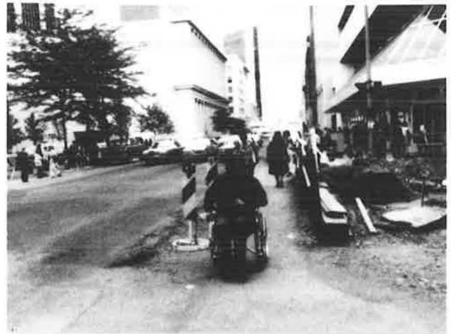
Figure 8. Inadequate separation and protection from vehicles endanger pedestrians' safety.
