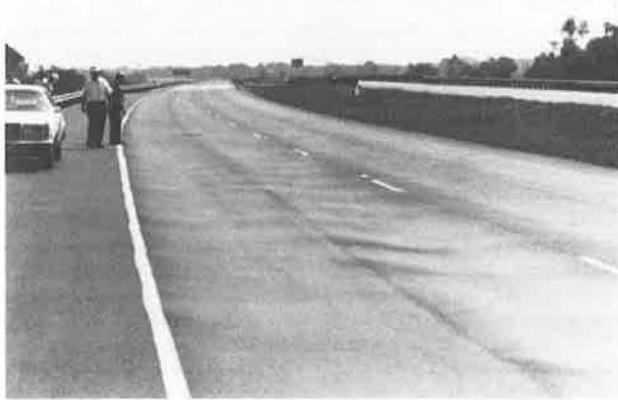
Figure 1. Typical rutting and corrugation distress.
