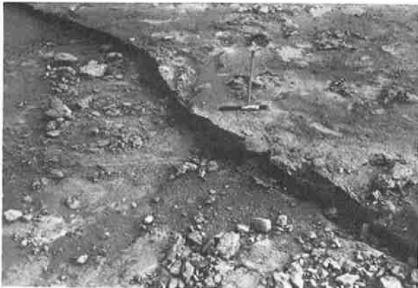
Figure 7. Stress relief expansion of saprolite from gneiss exposed in structural excavation.
