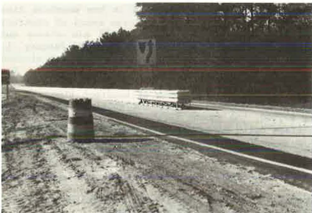
Figure 7. Crossover barrier and attenuator.
