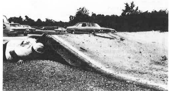
Figure 1. Blowup of concrete highway pavement in Ohio.
