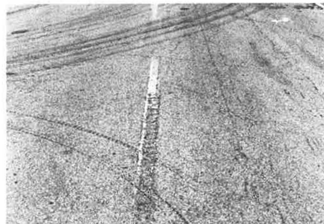
Figure 8. White premixed paint (centerline) still visible after 12 years of service.
