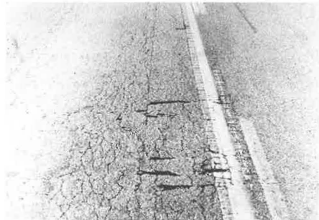
Figure 7. White premixed paint (centerline) after 12 years of service, shown between yellow lines.
