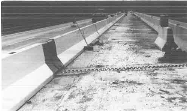
FIGURE 6 Pennsylvania Turnpike: Polymer concrete shells installed and awaiting placement of infill concrete. (Note the pour holes at the top of the barrier and the splice section to the right).
