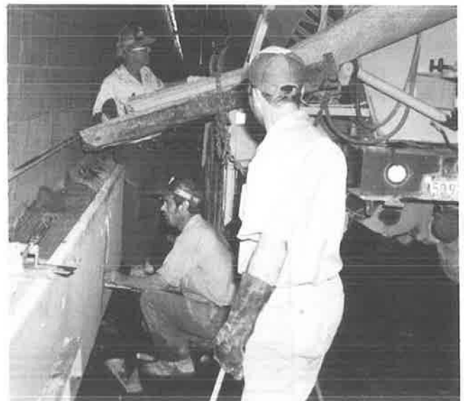
FIGURE 9 Sumner Tunnel, Boston: Work crew places conventional portland cement concrete with a superplasticizer additive between the polymer panel and the existing sidewall concrete.
