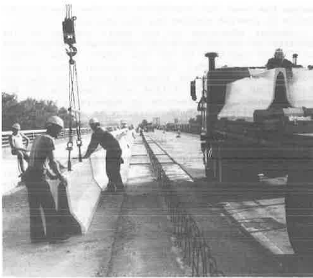
FIGURE 5 Pennsylvania Turnpike: Erection crew unloading polymer concrete shells prior to setting over reinforcing bars.
