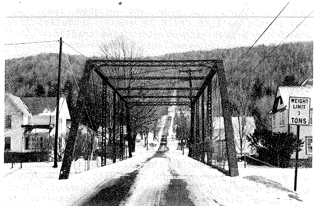
FIGURE 1 Coudersport bridge before rehabilitation.
