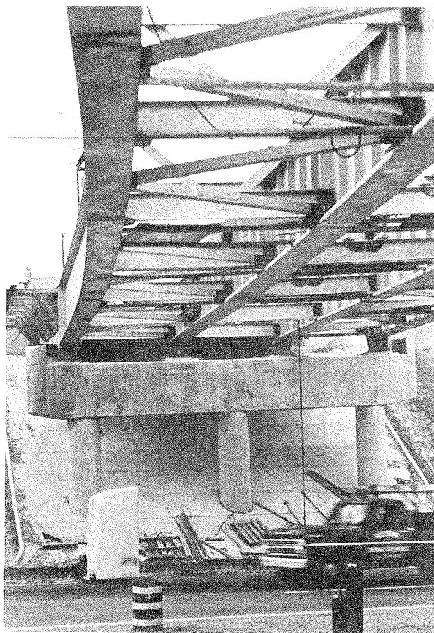
FIGURE 1 View showing curvature in the girders and design of diaphragms and lateral cross bracing.
