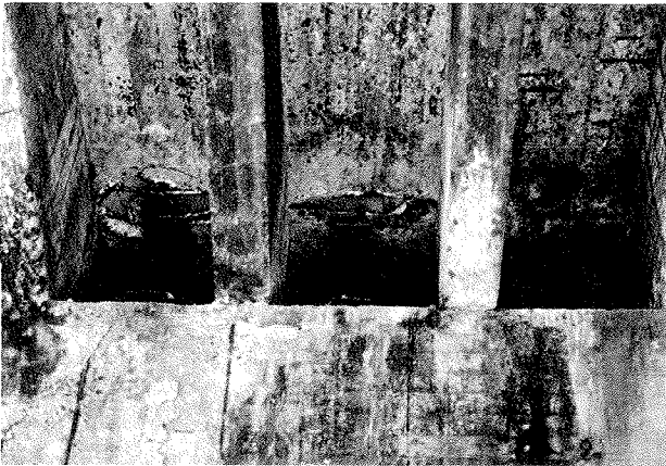
FIGURE 10 Holes in structural slab.
